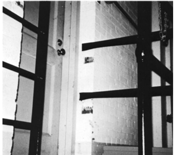
FIGURE 7.2 New guardrails. Some employers tore down their guardrails and rebuilt them 3 or 4 inches higher just to meet OSHA's standard in the early years of OSHA enforcement. Note the paint marks on the wall where the old guardrail had been attached. OSHA has since relaxed its rule somewhat.
