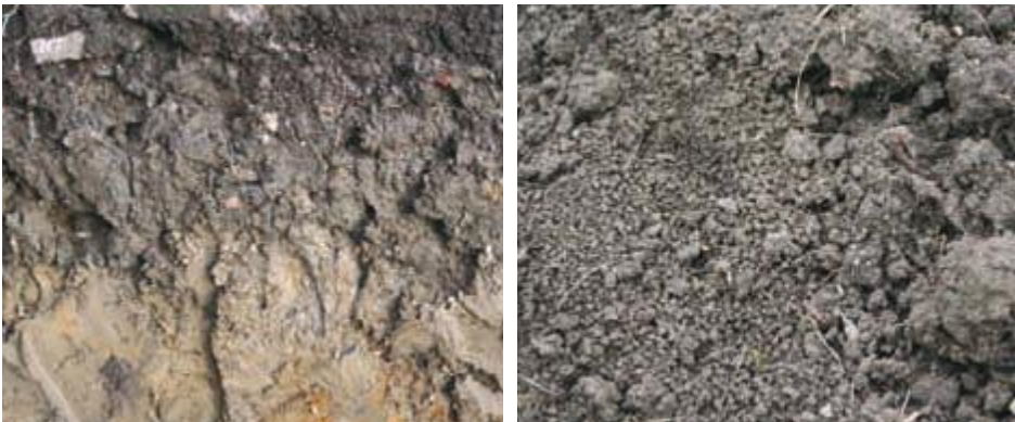
Left: The profile of the trench for building the conservatory – shows dark loam over clay. Right: Surface loam – shows how after frost you can make a tilth by knocking clods.
